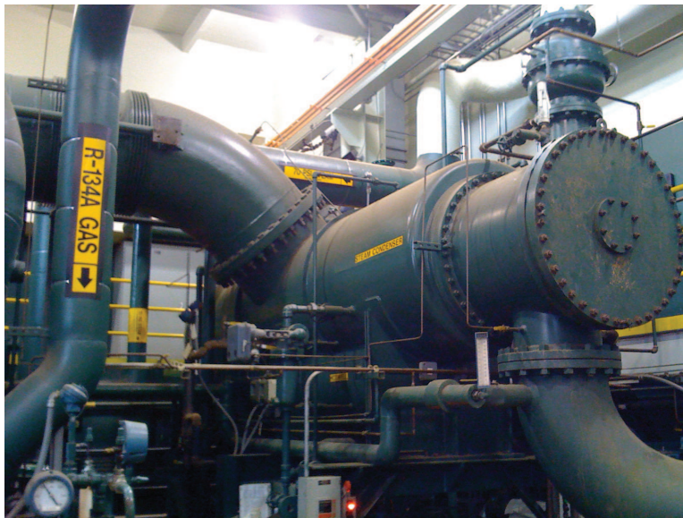
Figure 10.18: Chiller in the University of Notre Dame power plant, 14 June 2010.
