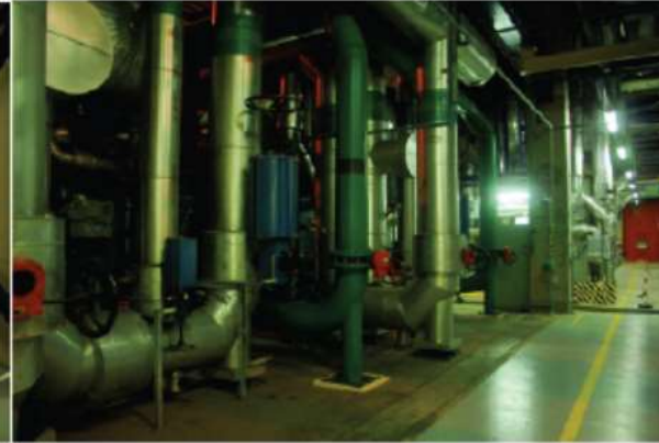
Internal cooling system for the GRC (compression chillers)
