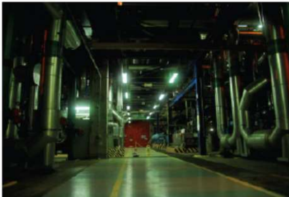
General view (far end, chillers cooling system pumps)
