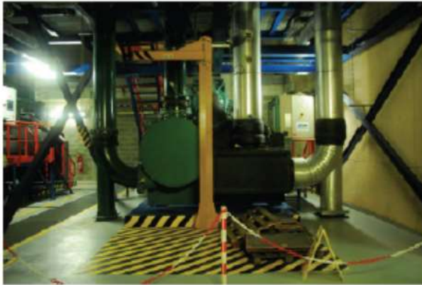
Absorption chiller (green – condenser; black – evaporator).
