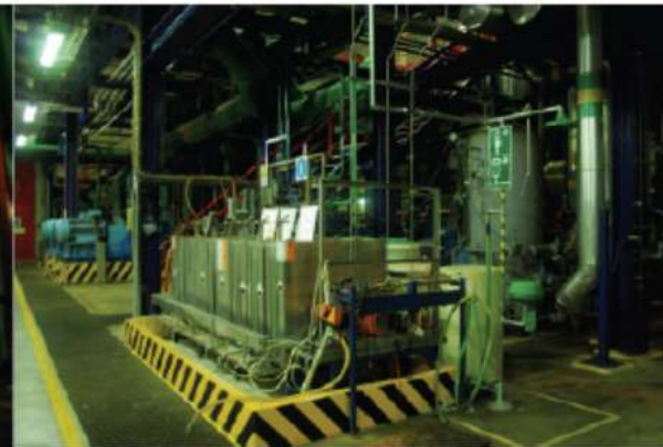
Water treatment station
